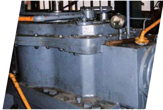
建國抽水擴建站 可動翼葉輪檢修 Jianguo pump station Examination for impeller
