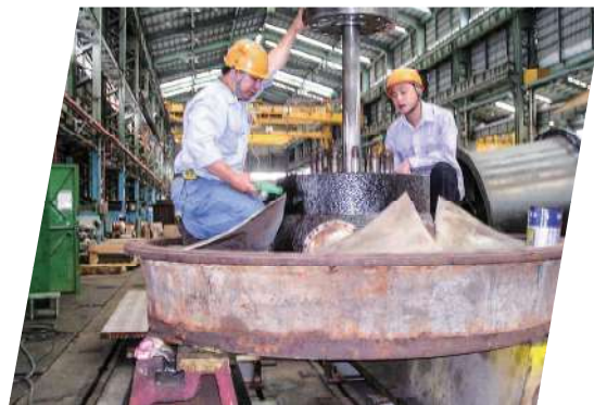
建國抽水站角齒輪減速機檢修 Jianguo pump station Examination for gear reducer
