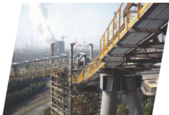
中鋼煉焦爐增設煤倉設備 CSC Coke Oven Plant Coal Bin & Conveyor
