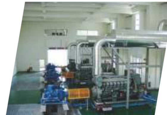
新生擴建抽水站 抽水機組現場安裝 Xinsheng pump station On-site installation
