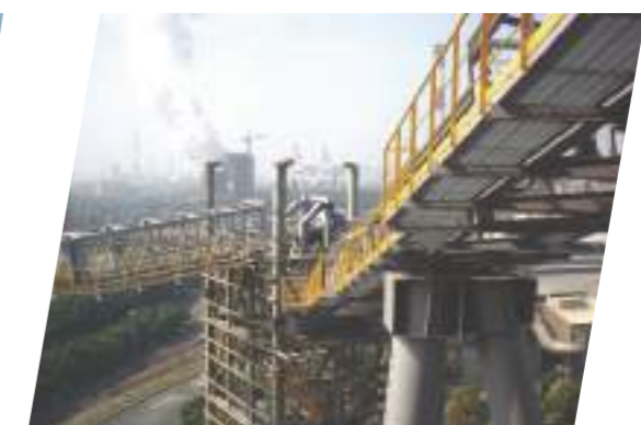
中鋼煉焦爐增設煤倉設備 CSC Coke Oven Plant Coal Bin & Conveyor
