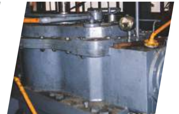
建國抽水擴建站 可動翼葉輪檢修 Jianguo pump station Examination for impeller
