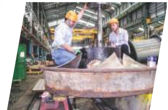
建國抽水站角齒輪減速機檢修 Jianguo pump station Examination for gear reducer
