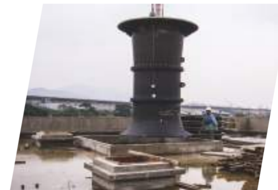
新生擴建抽水站抽水機組 下部組件現場吊裝 Xinsheng pump station On-site installation
